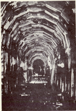
Interior of the South Park's Alpine tunnel, photographed in 1962. Eighty years after its construction, the redwood timbering still glistens solidly above the old rails. Much of the road-bed is under water, but in this stretch the rails are still above the water line. Photo courtesy of J. L. McClelland.
